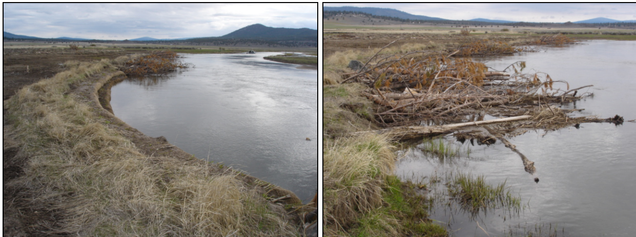
Figure 4-6. Example bioengineering (left) and engineered log jams (right) on the Sprague River. Bioengineering and log jams provide bank stability and diverse aquatic habitat. Over time, the willows planted in the soil lift will form a dense willow thicket.
