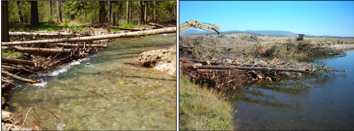
Figure I-7. Example ELJs constructed on a moderate gradient alluvial stream in Idaho (left) and on the Sprague River near Beatty, Oregon (right).
