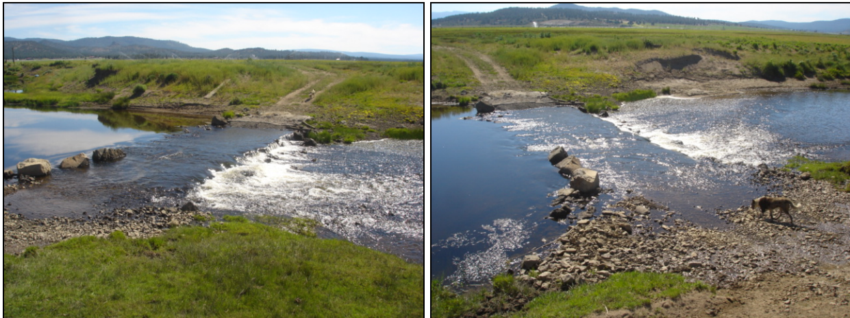
Figure 5-6. The Kronenberger crossing likely creates a fish passage barrier during baseflow. These picture taken in June 2007, capture the structure during the declining hydrograph.
