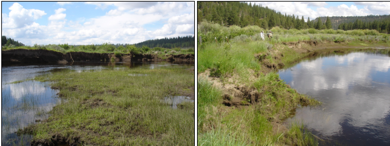
Figure B-22. Example bank conditions in Reach 3. Severe bank erosion from Station 97+00 to 99+00 (left) suggests continued down valley meander migration.
