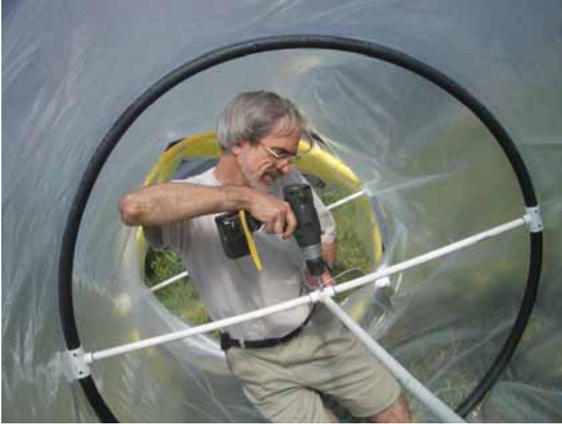
Figure 16. Assembly of larger enclosure. Note drilling of hole in central fitting and vertical connector pipe for cable tie. Circular spreaders were preassembled.
